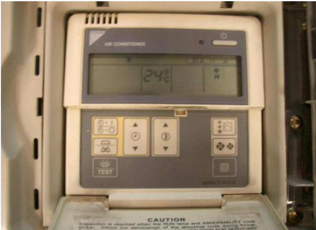
Figure 4-5: The control unit of VRV system in BYTE building
