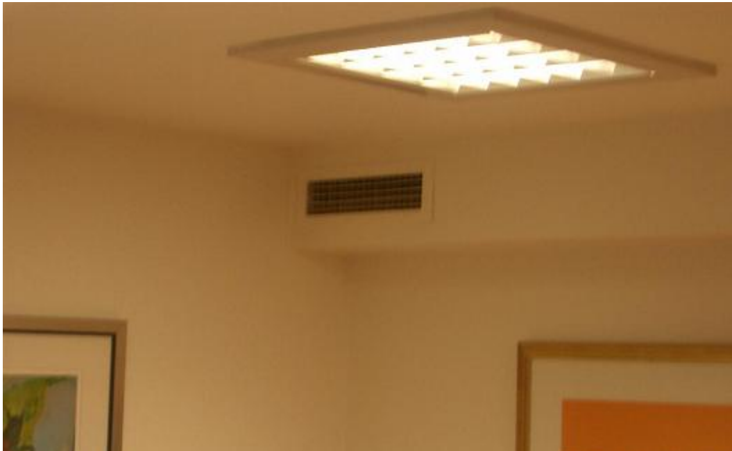
Figure 4-7: The electric lighting system of BYTE building.
