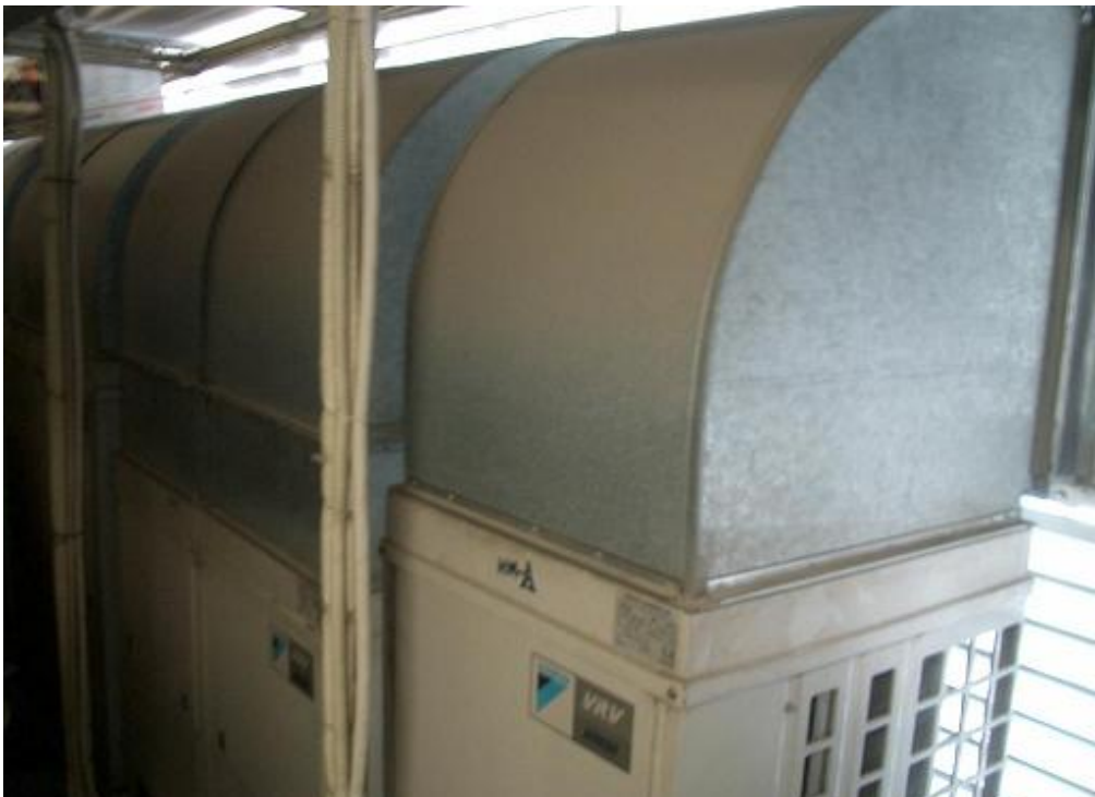
Figure 4-4: The outdoor units of the VRV system in BYTE building
