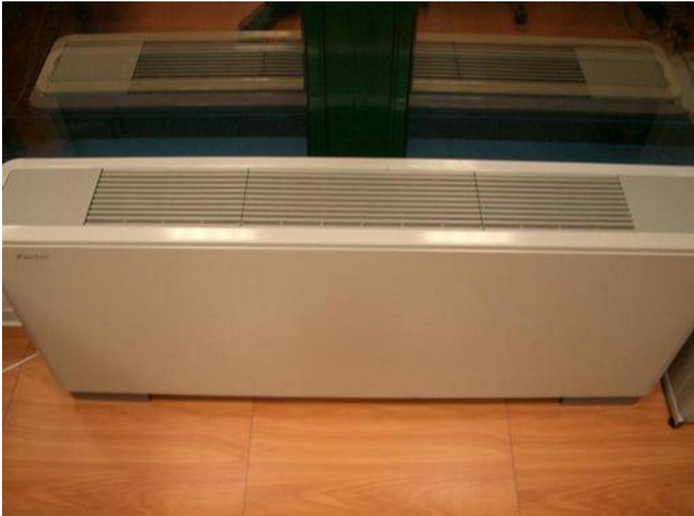
Figure 4-3: Local unit of VRV System in BYTE building
