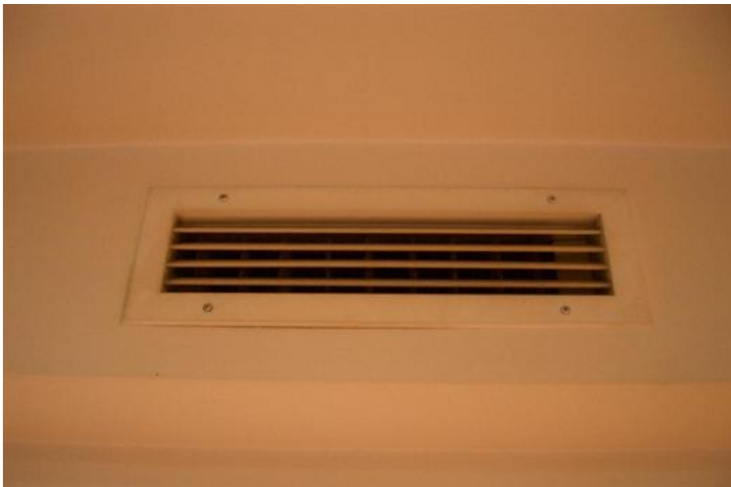
Figure 4-6: The air vents of the ventilation system
