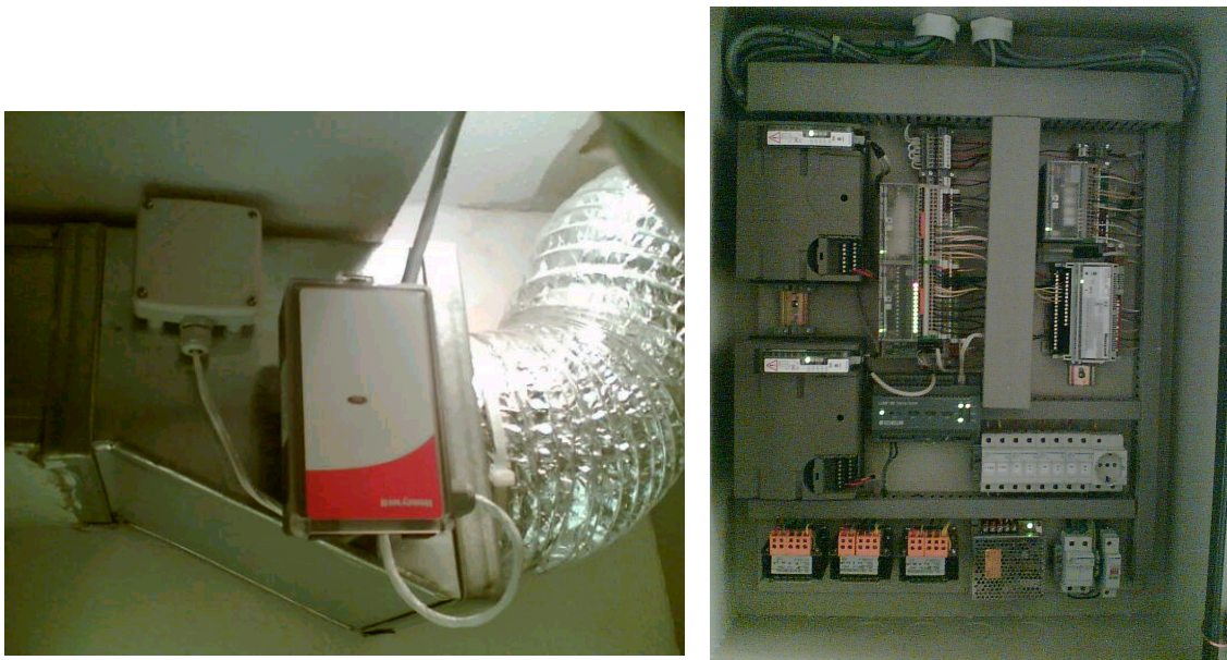
Figure 4-9: The BMS hardware
